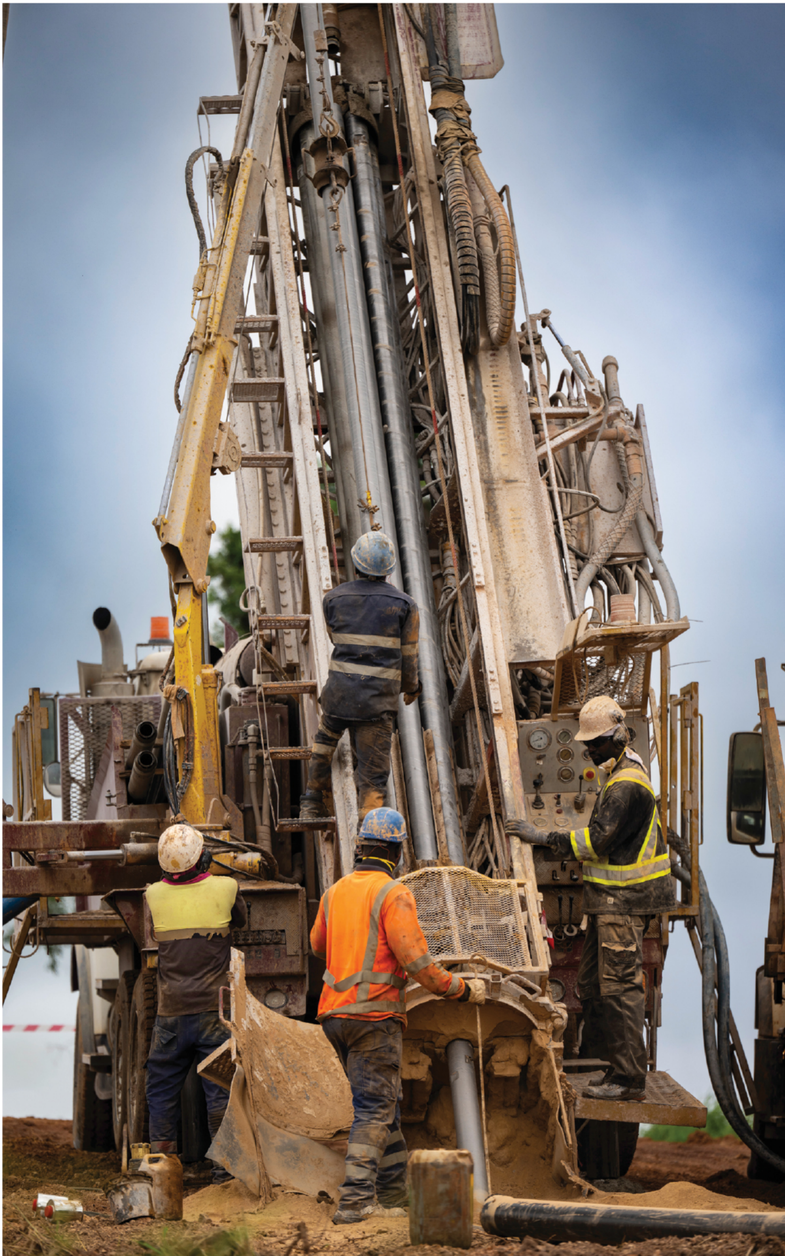
↑ A drill rig operating at the La Debo project in the south of Côte d'Ivoire
